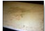
Replaced or re-laminated top
